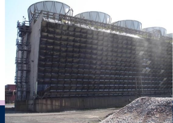
Mechanical-Draft Cooling Tower. Source: Tetra Tech
