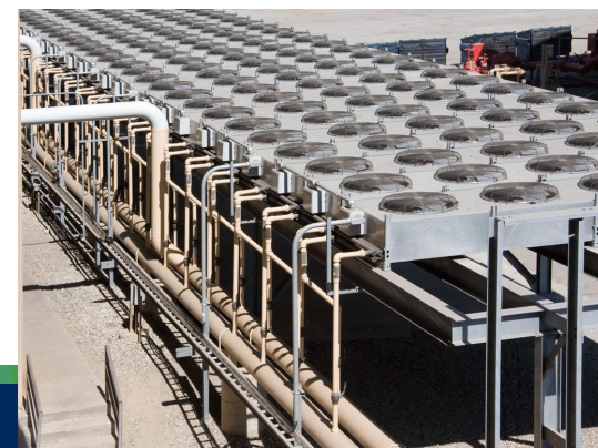
Air Cooling Fan-Array. Source: EvapCo
